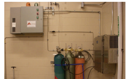
Methane to Power
