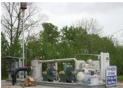
Flare System St Landry, LA
